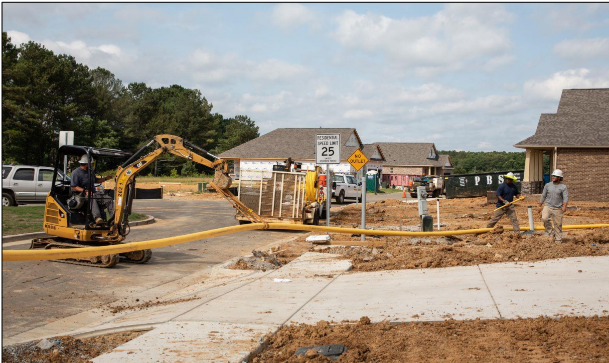
Natural gas customers continue to increase by around 3% annually. Shown above is an HU crew installing residential gas lines.
